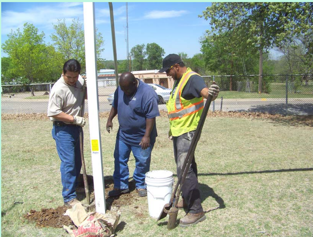
Public Works personnel recently assisted at Harlean Beal Elementary by installing playground equipment. Pictured are Supervisor Roberto Duenes, Albert Harris and Ed Perez.
